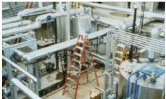
Completely shop fabricated equipment skids can significantly reduce field installation cost and schedules.
